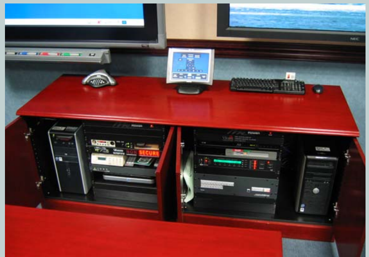
Equipment credenza with Middle Atlantic sliding rotating equipment racks
