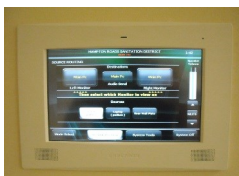
Crestron custom control panel provides simplified room operation for end-users
